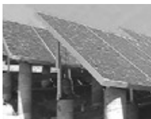
New BP Solar 160 watt modules with MC connectors made this a low-labor installation.
